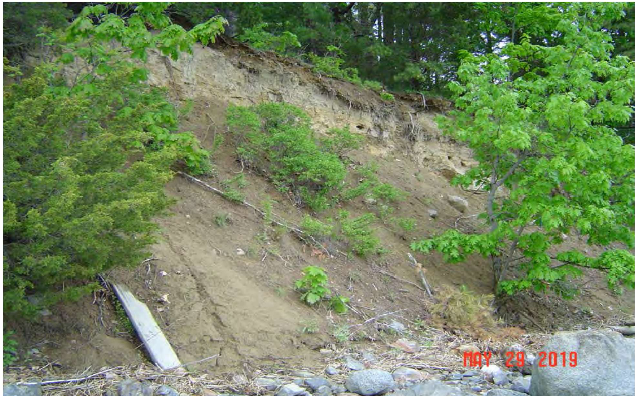
Image 3 – Looking northerly from flag C20± at bank erosion along the 'C' line in Newington. (©Jacobs 2019)
