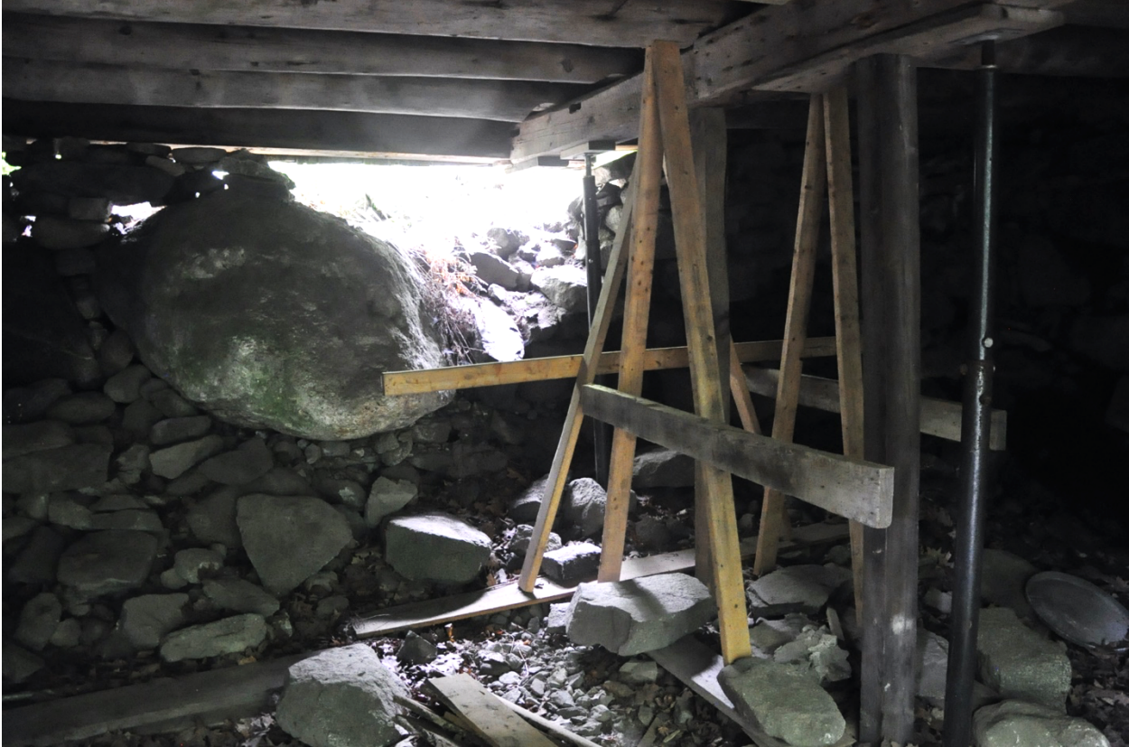
Erosion of the southwest foundation wall by stormwater runoff from Mill Road (photo taken from under the structure)
