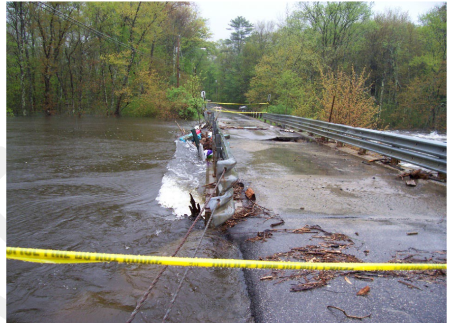
Wiswall Bridge during May 2006 Flood Event (Photo Credit: Durham Hazard Mitigation Plan)
