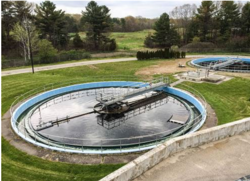
Clarifying tank at wastewater center (Photo Credit: Town of Durham)
