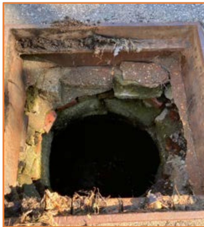
Dennison Road – example of deteriorated barrel block constructed drainage structure to be replaced with precast structures
