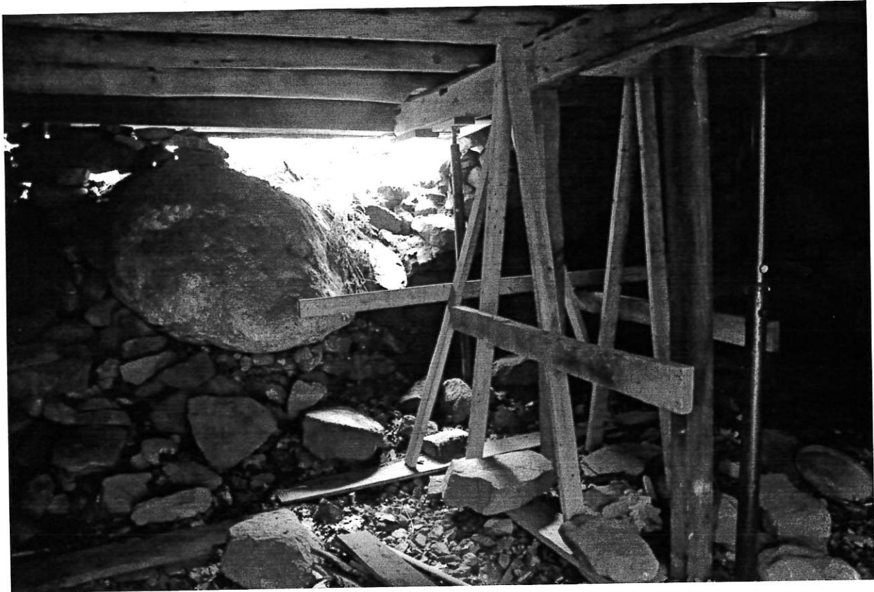
Erosion of the southwest foundation wall by stormwater runoff from Mill Road (photo taken from under the structure)
